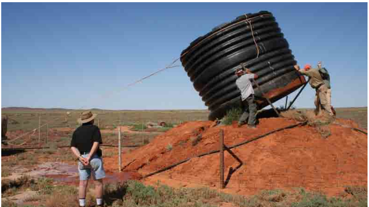
Volunteers relocating a water tank at Witchelina in December 2010. Photo: Hunting and Conservation Branch of the Sporting Shooters Association Australia.
