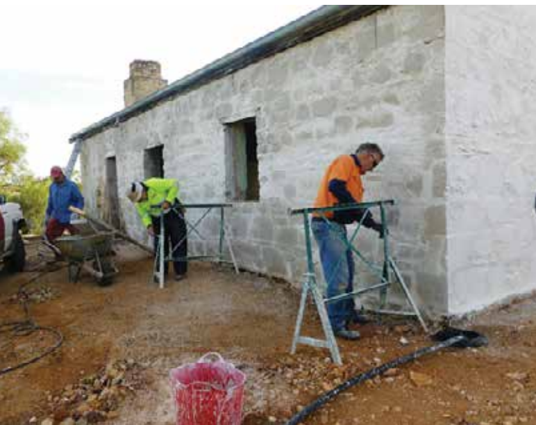
Hard at work: Restoration of the original shearers' kitchen and dining room building at Witchelina.
